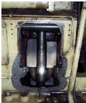
Damage to a $ 7 million generator in East Timor from poor maintenance
